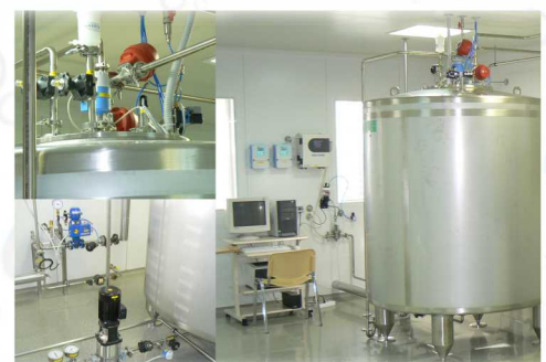
Hygienic pharmaceutical water storage and distribution system
