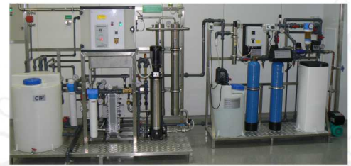
Pharmaceutical "Purified water" purification system in a Pharmaceutical plant
